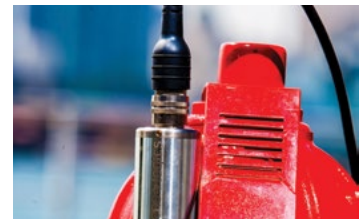
STEP 2: MOUNT TWO SENSORS OUTSIDE OF A SELECTED PIPE ON AIR VALVES, FIRE HYDRANT OR OTHER EXISTING APPURTENANCES.
